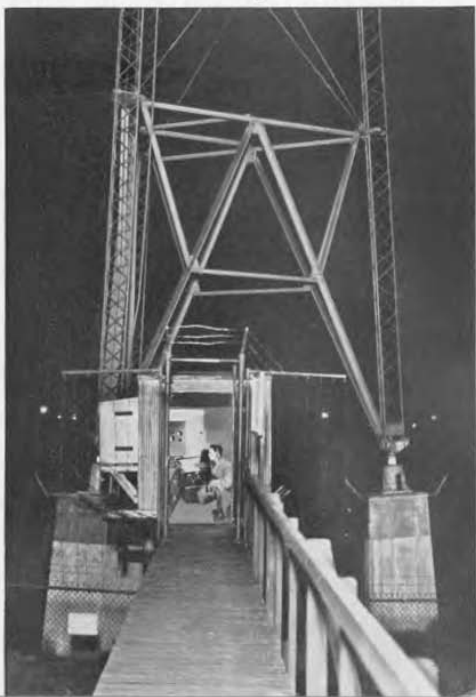
FIGURE 1. Measuring the impedance of an antenna tower as seen from the "dog house" at the base.
